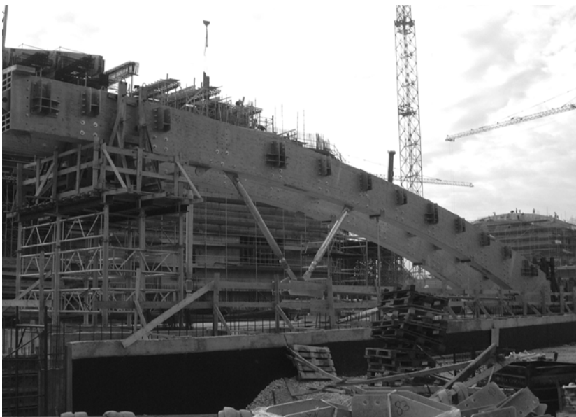
in order to assemble the whole truss a temporary tower has been used: the total weight of half truss being kg. 27000 (beam G11)
