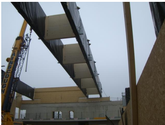
Illustration 7: Eton Manor sports facility. Installation of main beams. Image copyright PJ Steer.
